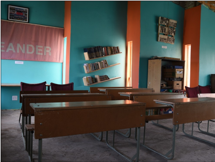
We painted the inside walls of our new building and we have almost completed the outside plastering.
